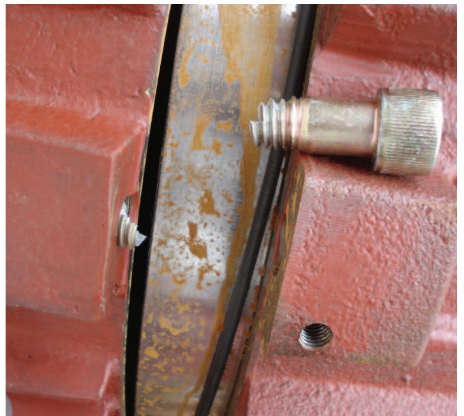
A Flameproof Enclosure is only as strong as its fasteners. Do all those installing, inspecting and maintaining realise the need to use only the fasteners specified by the manufacturer?
