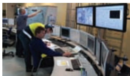
In the control room all gas flows throughout the plant are closely monitored.
