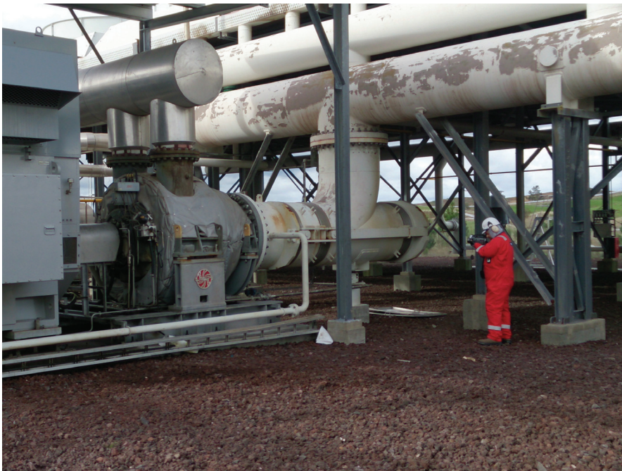
Small leaks can become big ones, that is why it is important to be able to detect them in an early stage.
