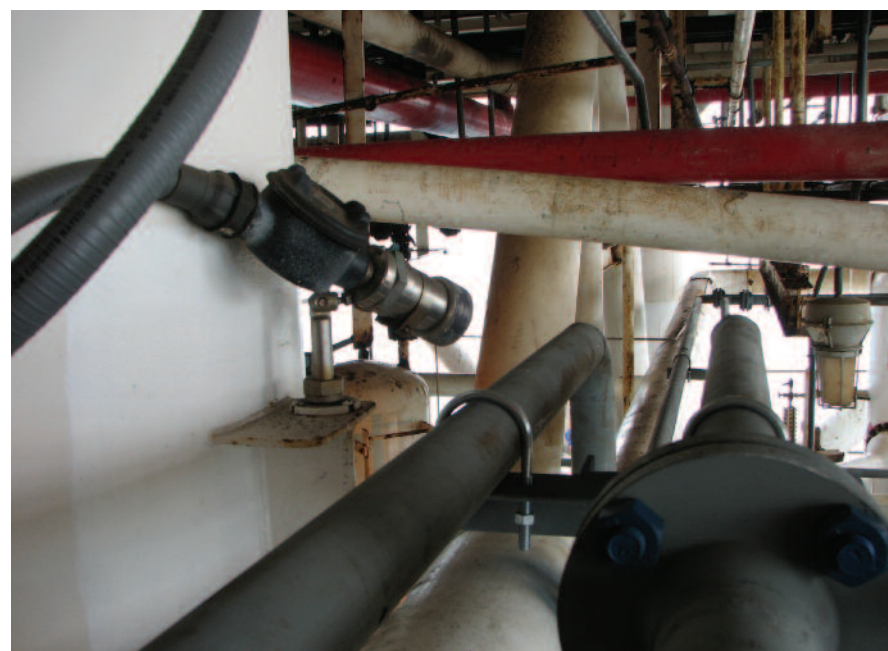
Figure 3. Flame detector view is blocked by obstructions.
