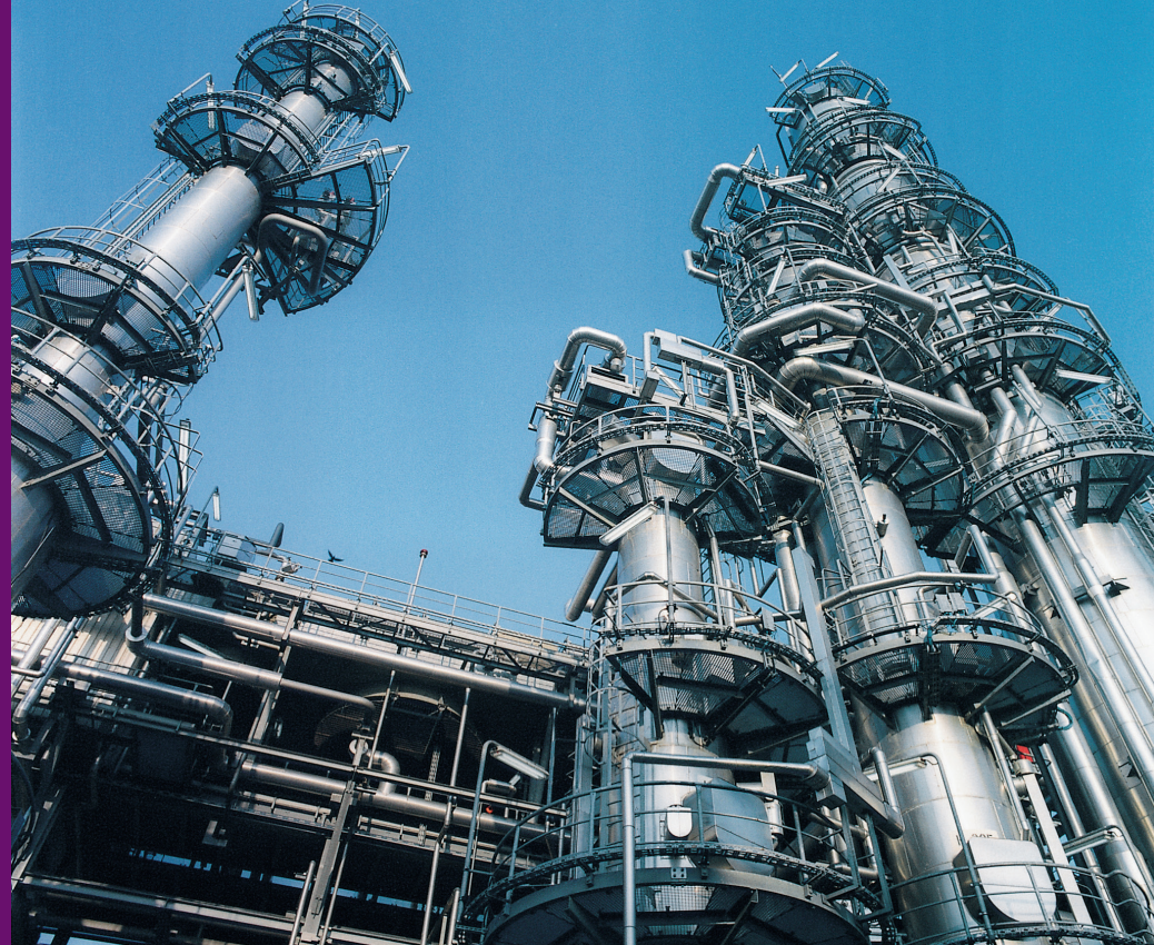
Typical distillation towers - A significant application field for process gas chromatographs © Siemens AG 2022, All rights reserved
