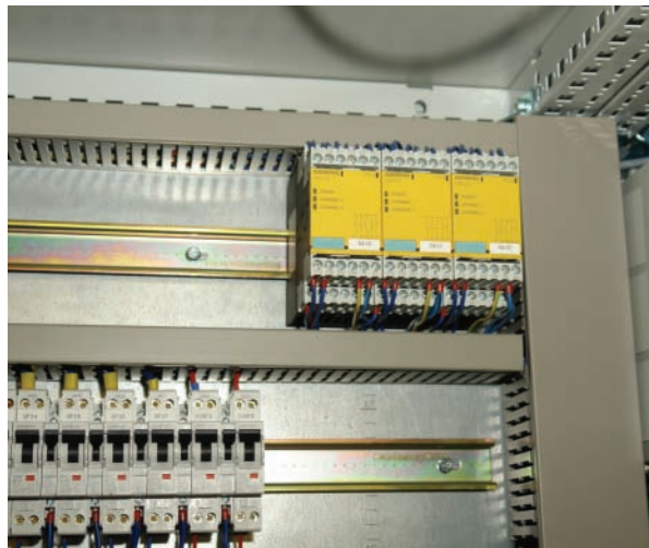
Figure 6. The assembly of three different safety circuits via 3TK28 safety relays by Siemens ensures that an EMERGENCY-STOP does not shut down the entire plant. In the biodiesel plant, this has proven extremely practical over the course of time.
