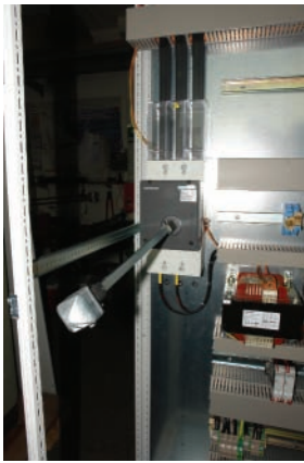
Figure 3. The Sentron 3VL molded-case circuit breaker is available up to 1,600 A. Thanks to its modular design, it can be easily adapted to individual requirements.
