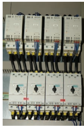
Figure 4. As a "material-sparing" alternative to conventional star-delta circuits, soft starters offer valuable services for pumps and agitators. In addition, the 3RW30, the most basic starters of the Sirius range by Siemens, are comparable to standard feeders in terms of prices.
