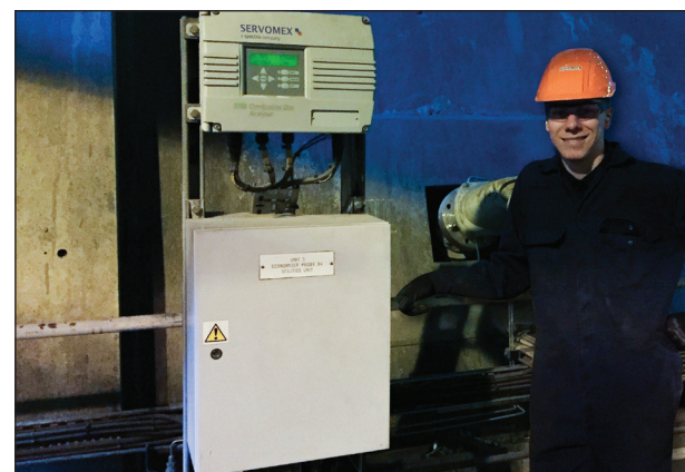
A FluegasExact 2700 installation – this provides measurements to control combustion reactions
