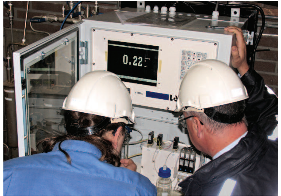
Figure 4: Commissioning and start-up of a QuickTOCpurity TOC analyser
