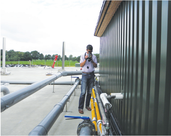
Explosion protected areas can be investigated from a safe distance with the FLIR GF320.
