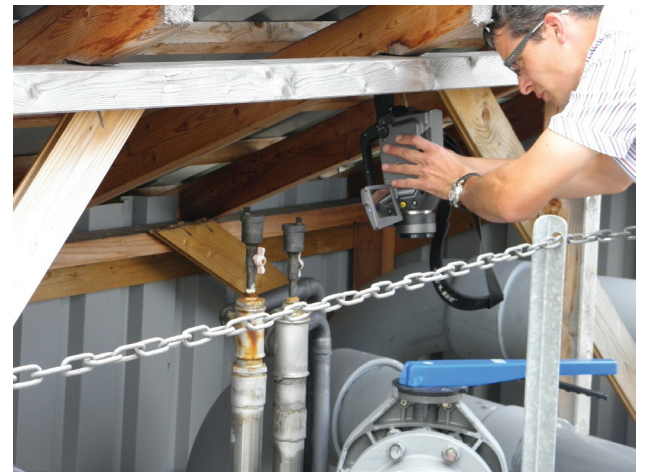
Engineer Ibeling van Lessen looking for gas leaks, which is possible from a safe distance and unusual angles using the FLIR GF320.
