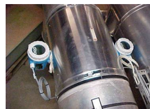
New twin sensor gas meter
