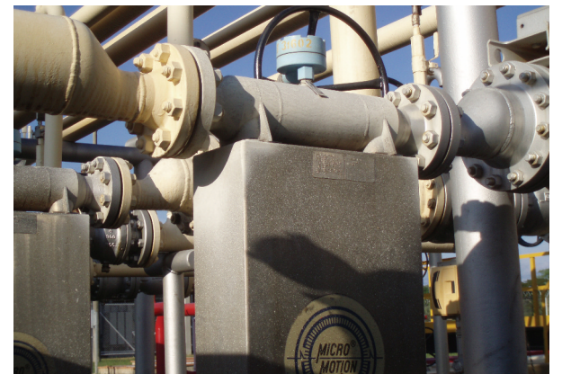
Poor design of LPG meter installation
