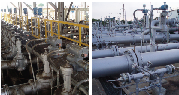
Crude Oil inlet (American PD meters shown)
