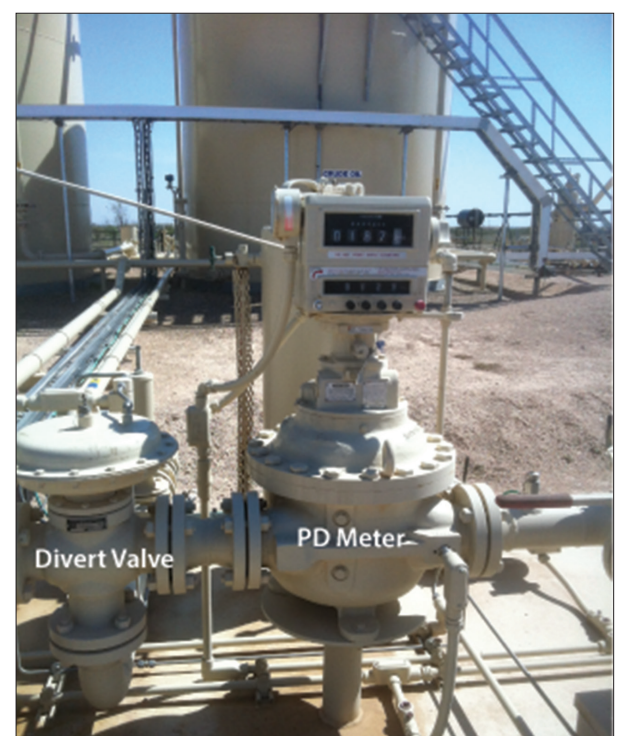
Meter Portion of LACT Unit
