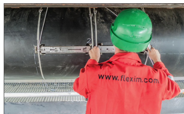
On the heated pipeline for refinery residue products, the ultrasonic transducers are integrated into the insulation.
