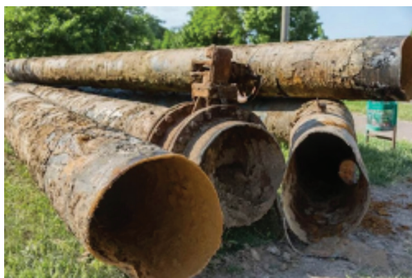
Figure 1: When exposed to the elements and not properly maintained, iron pipes can corrode away leading to having to replace the pipes.
