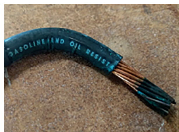
Figure 1: Corroded Copper Wires [8]
