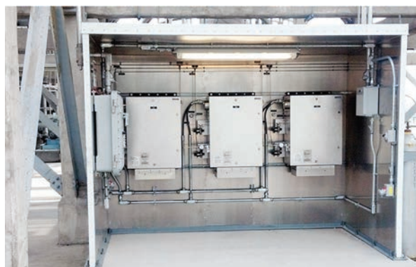
Three-stream process system in three-sided shelter.
