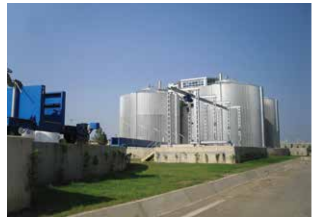
Waste water treatment plant in Turkey
